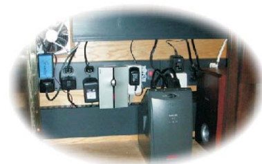
90 DEGREE INDUSTRIAL POWER STRIPS AND CABLE TRAY
